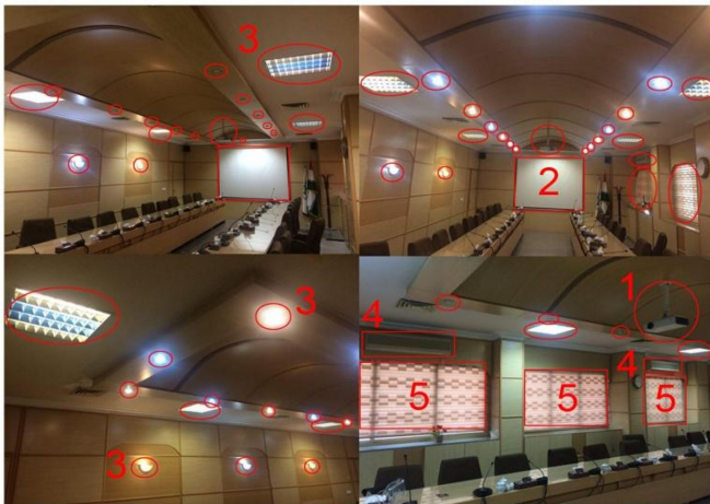
Fig. 3. Conference room was used as the more complex room. The interactable devices in the conference room are circled: 1) video projector; 2) electric projector screen; 3) different types of lamps; 4) air conditioners; and 5) electric roller blinds.
