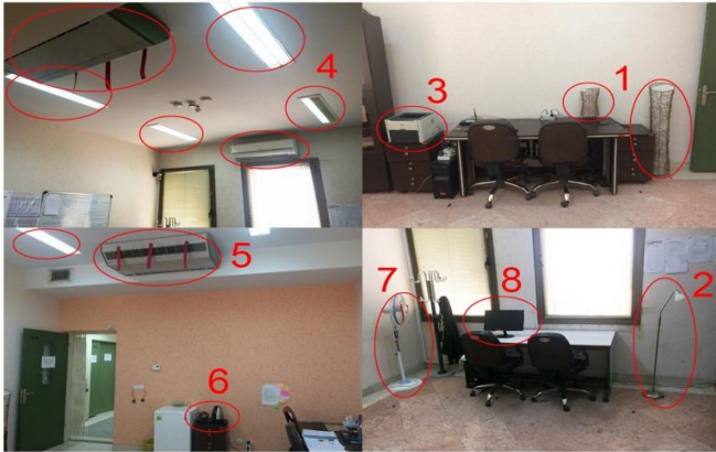
Fig. 2. AmI Lab was used in the experiment as the less complex room. The marked objects were interactive: 1) standing light; 2) lampshade; 3) printer; 4) ceiling lights; 5) air conditioner; 6) tea maker; 7) standing ventilator; and 8) monitor.
